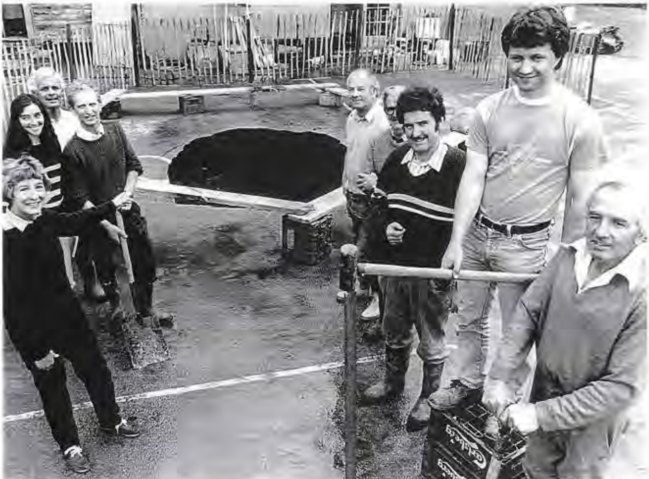
When the rains came—1987 Collapsed culvert in the School Yard
